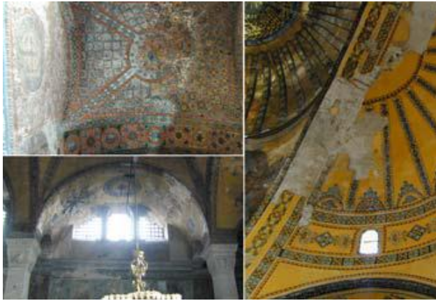
Fig. 18. Details of the state of preservation of the surfaces inside the building.
