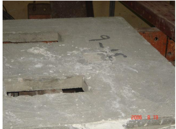
Fig. 17. Crushing of concrete at the top surface of one of the tested slabs after failure.
