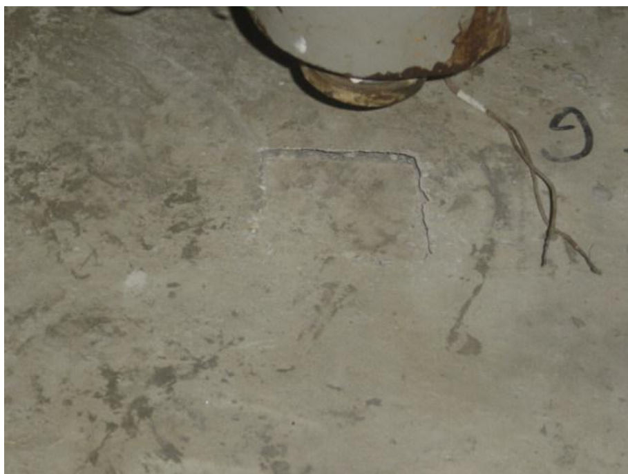
Fig. 9. Top view for one of the tested slabs after failure.
