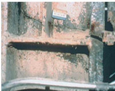
Fig. 1. Example of overloading induced cracking in steel frame joint.
