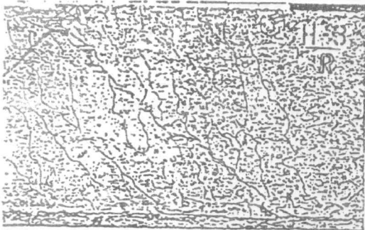
Figure 4. Yield-line and crack pattern at failure, (H-3), B/L=0.5, \phi=45^\circ .
