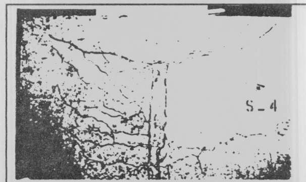
Figure 6. Tension side of (S-4) after failure.
